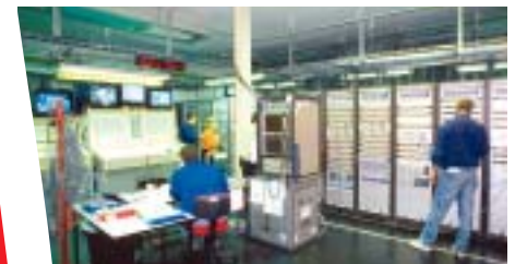
Industrial processes; programmable logic controllers, speed control processors, etc.
