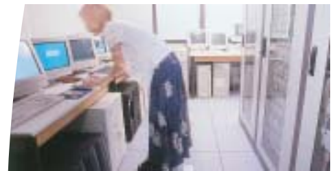
Servers and data storage, active network devices, etc.
