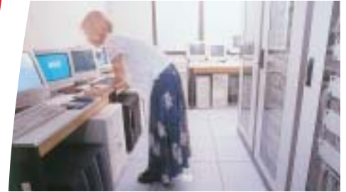
Data servers, storage units, backup devices, routers, etc.
