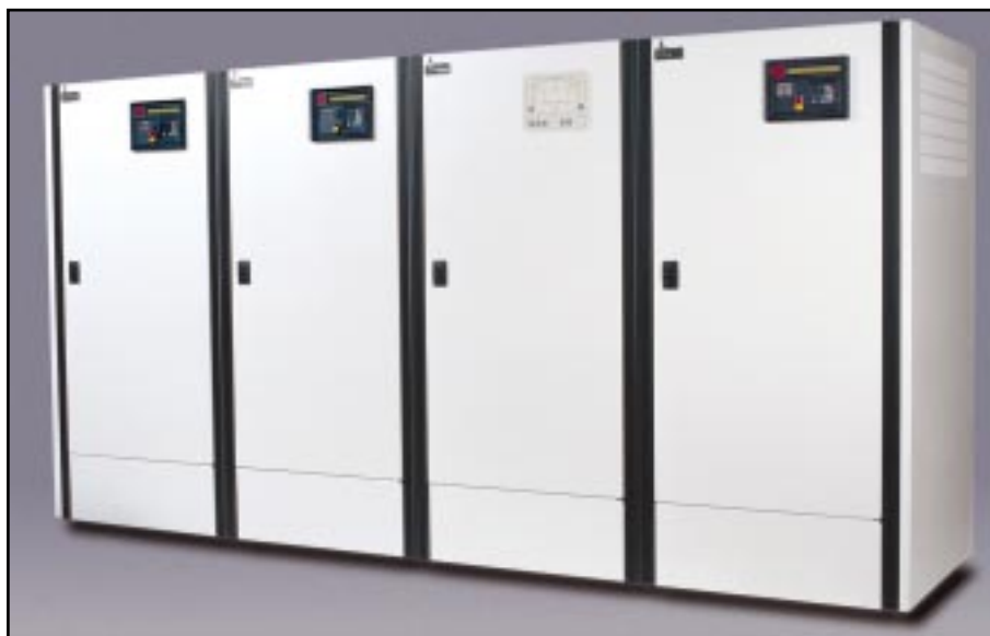
A static transfer switch integrated into the PDM increases system reliability and flexibility.
