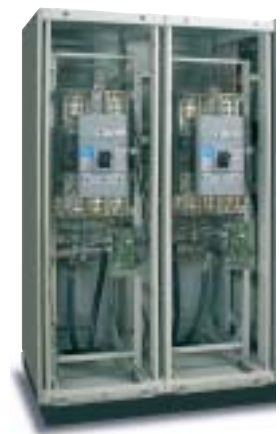
Battery Breaker Boxes without panels
