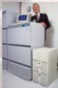
Telecom equipment at Ricard International
