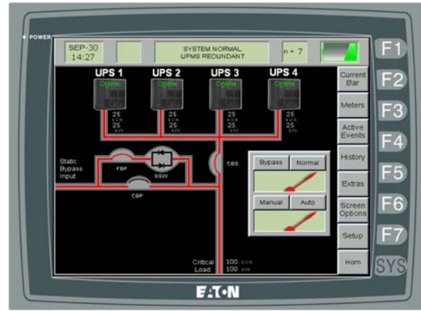
LCD display showing online system with closed system output breaker (CBS), open system bypass breaker (CBP)
