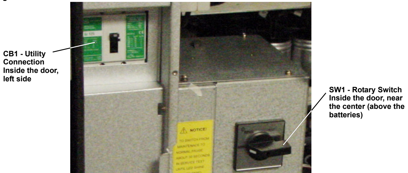
Figure 14 Power switches - 10kVA NX
