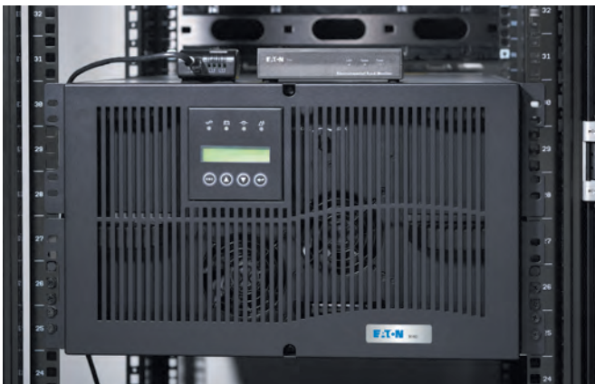
Eaton 9140 UPS with ERM and Environmental Monitoring Probe.
