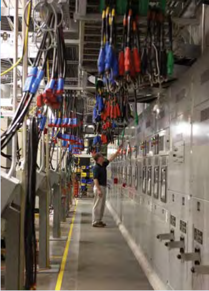
Eaton's Witness Test Centers allow you to see your large multi-module system tested before it's deployed.
