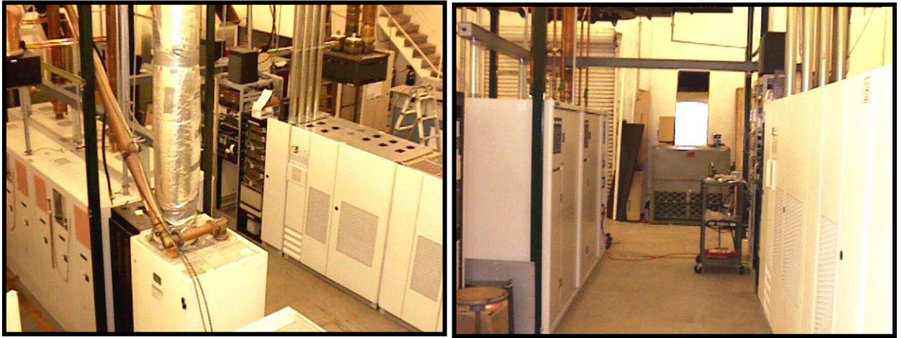
Figure 11- MGE EPS 6000 UPS supporting an IOT transmitter. This site has experienced numerous crowbars with the UPSs managing the fault without incident.
